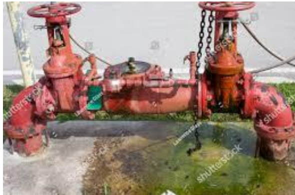
Figure 3-3 Packing Leaking of a Gate Valve
