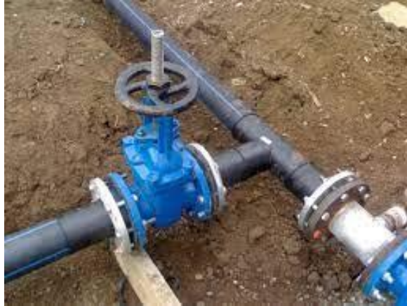
Figure 3-4 Gate valve fitted on a pipeline
