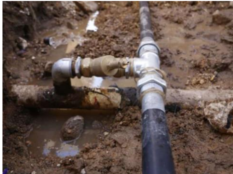
Figure 4-3 Pipe leaking underground
