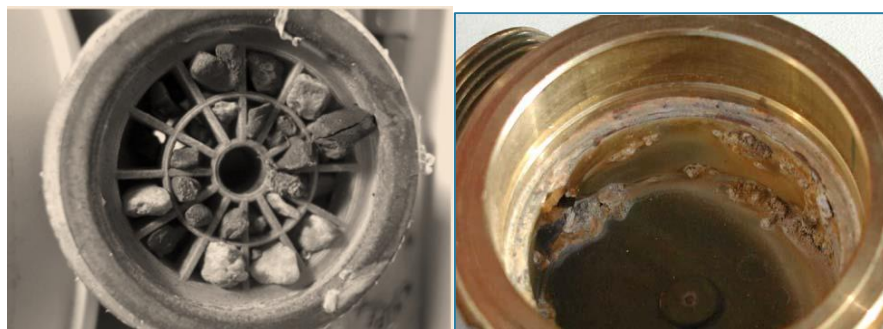
Figure 9-7 partial clogging caused by suspended particles and Lime scale
