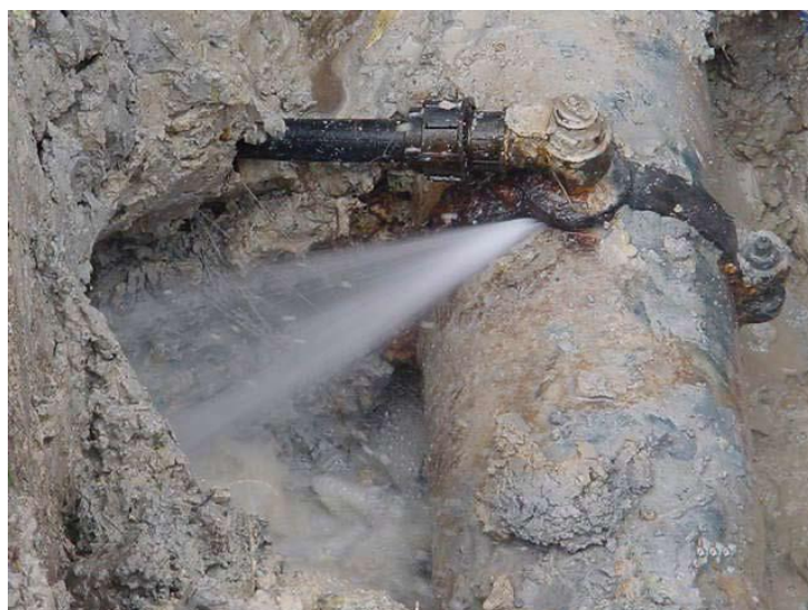
Figure 8-2 Small leaks go undetected
