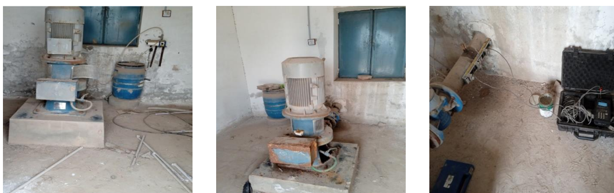
Figure 5: Sample pictures from field audit of pumpsets
