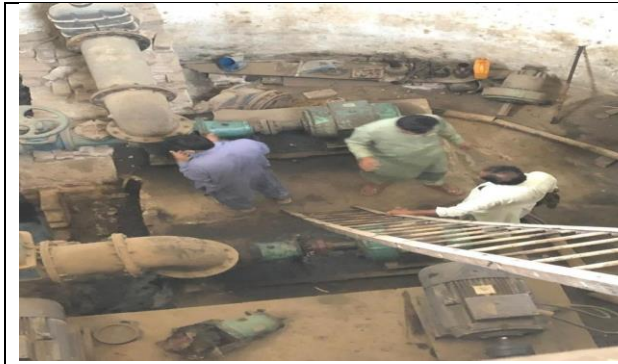
Balwant Pura disposal Pump House before installation of Sullage Pumping Units (5 Cusec)
