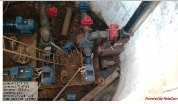
Balwant Pura Disposal Pump House after installation of Sullage Pumping Units (5 Cusec)
